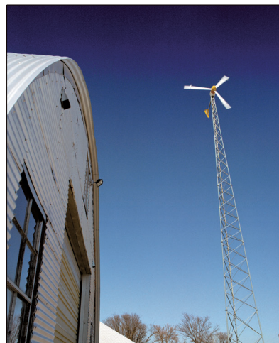
Grid-Connected Small Wind Turbine
