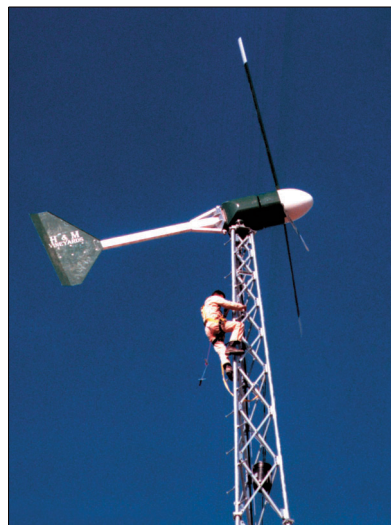
Small-Scale Wind Installation
