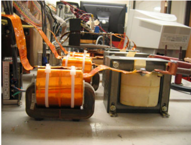
Figure 6.6: Filter inductors at one converter terminal
