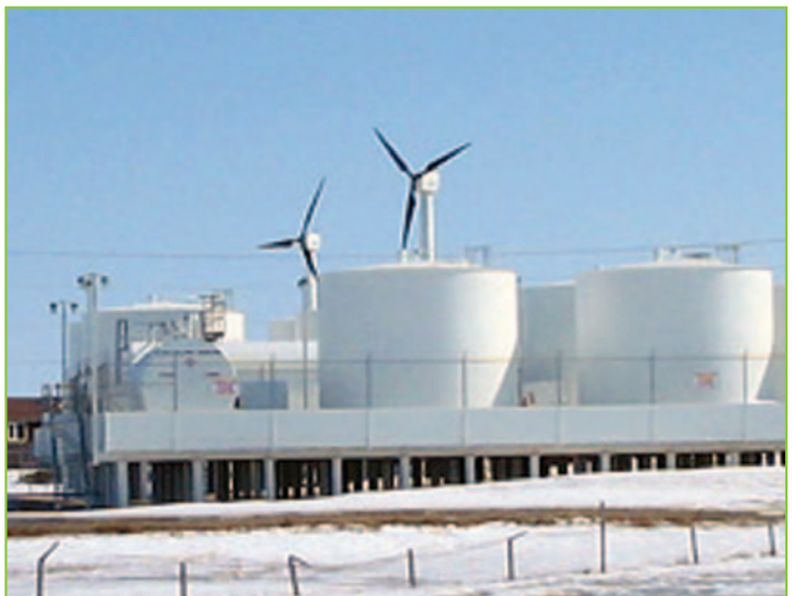
Two of three wind turbines can be seen over the bulk fuel tanks of the Kasigluk Power System. Ian Baring-Gould/PIX16097.
